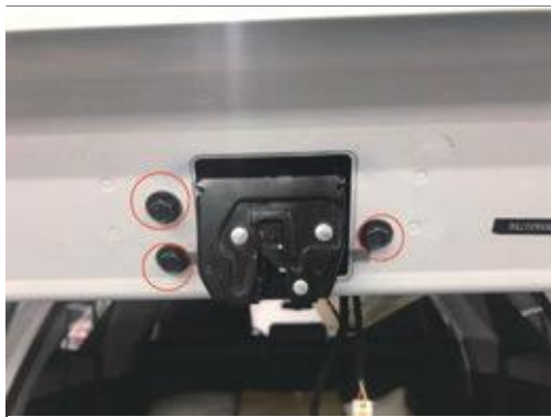
13. Remove the original locks and install the electric suction locks of our company, and fix them with screw and flat washer.
